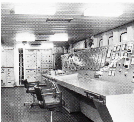
Maskinens kontrolrum. The engine control room.
