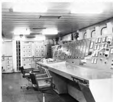
Maskinens kontrolrum. The engine control room.
