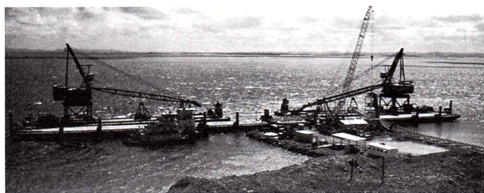
Den fremtidige udskibningshavn under bygning. The new port begins to take shape.
