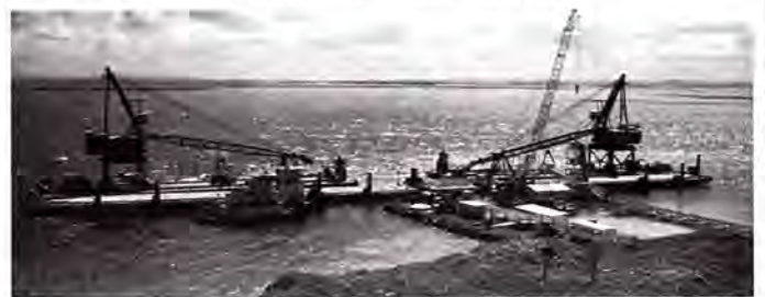
Den fremtidige udskibningshavn under bygning. The new port begins to take shape.
