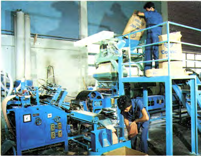
Special grades of Polyvinyl Chloride resins are being used for the production of battery separators at the Plant of Associated Battery Manufacturers Ltd.
